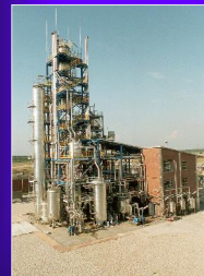
Hydrogen Peroxide plant
